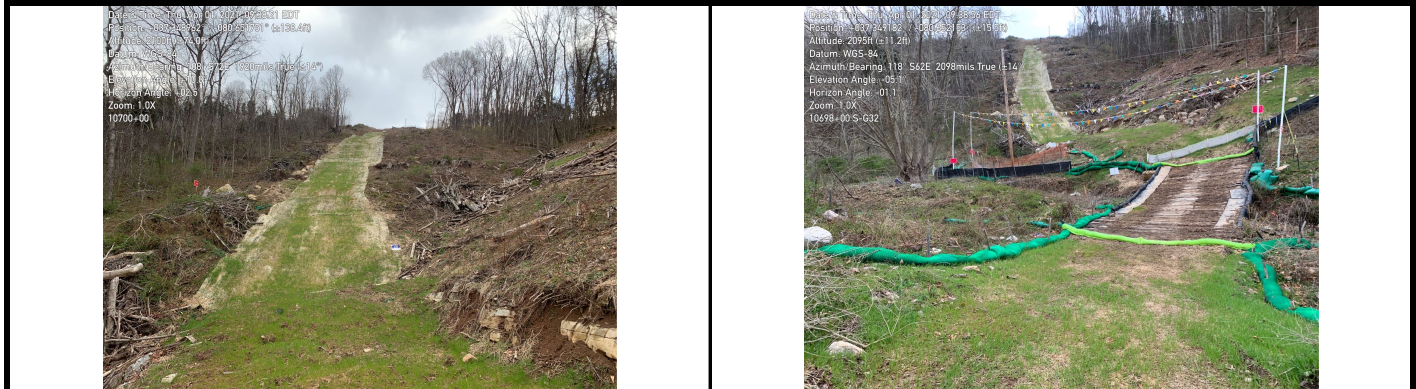
GPS Location See photo for GPS location. GPS Location See photo for GPS location. Field Station# 10700+00 Field Station# 10698+00 Pic 3 Desc. Steep slope stabilized with ECB. Pic 4 Desc. Sensitive resource buffer in place at stream S-G32.
