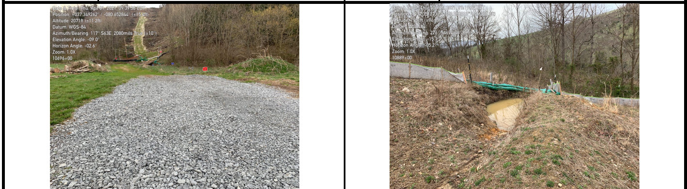
GPS Location See photo for GPS location. GPS Location See photo for GPS location. Field Station# 10696+00 Field Station# 10889+00 Pic 5 Desc. RCE in place at Buffalo Anklets Road. Pic 6 Desc. Triple stack 12 inch CFS in place at waterbar outlet.
