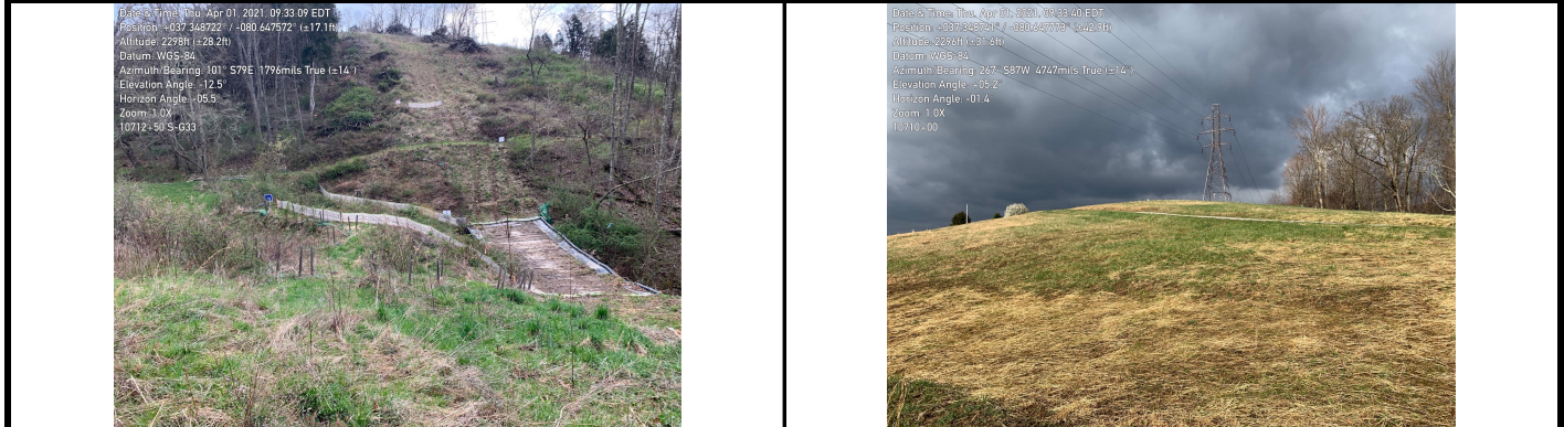
GPS Location See photo for GPS location. GPS Location See photo for GPS location. Field Station# 10712+50 Field Station# 10710+00 Pic 1 Desc. Sensitive resource buffer in place at stream S-G33. Pic 2 Desc. ROW stabilized with natural vegetation growth.
