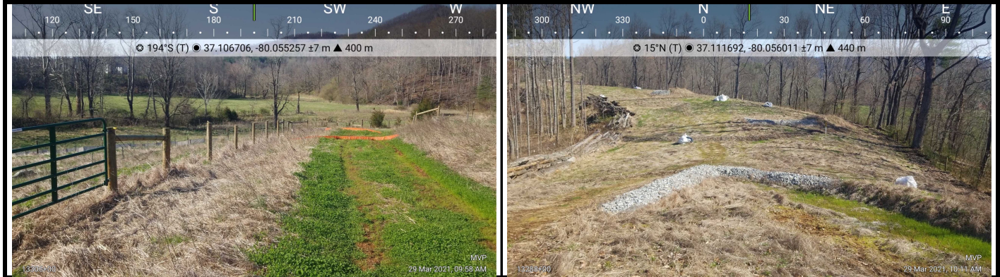
GPS Location See photo coordinates. GPS Location See photo coordinates. Field Station# 13306+00 Field Station# 13288+00 Pic 3 Desc. ROW stable with vegetative cover across LOD. Pic 4 Desc. ROW stable with vegetative cover across LOD.
