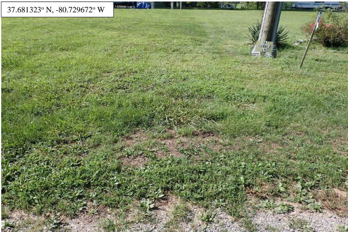
Photo Type: Left Side of AR Location, Orientation, Photographer Initials: Left Side of Access Road, AK/RA/TA
