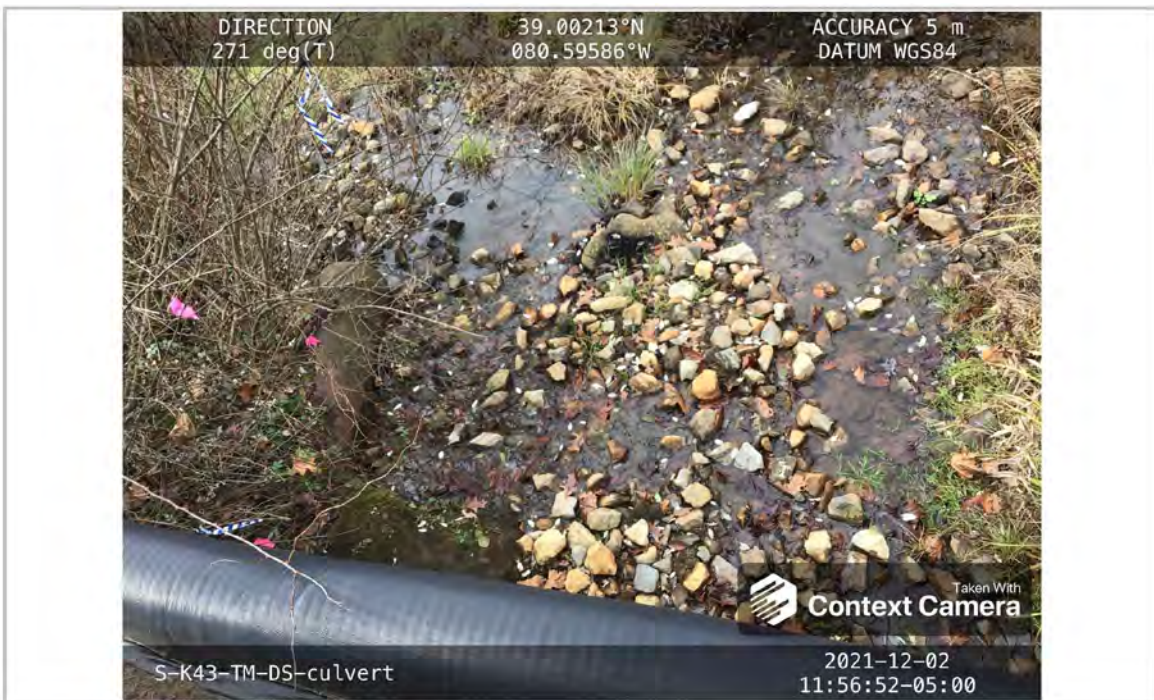
Photo Type: Downstream View Location: 39.00213, -80.59586 Photo Orientation: W (271 degrees) Stream Type: Plane bed
