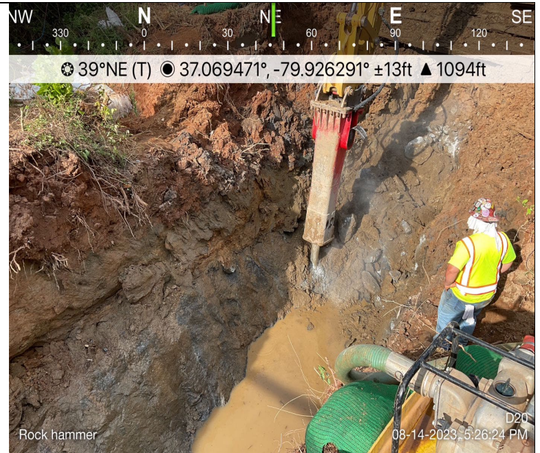
Photo Description: Removal of bedrock in pipeline trench with rock hammer attachment.
