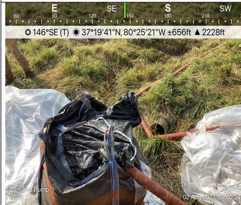
Photo Description: Existing flume and material to be used staged within buffer.
