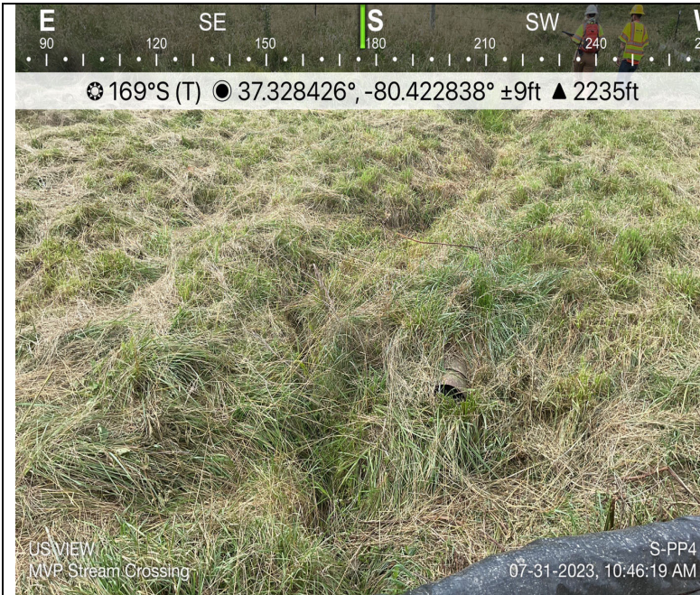
Photo Description: Existing flume in S-PP4. Not conveying water at time of photo.
