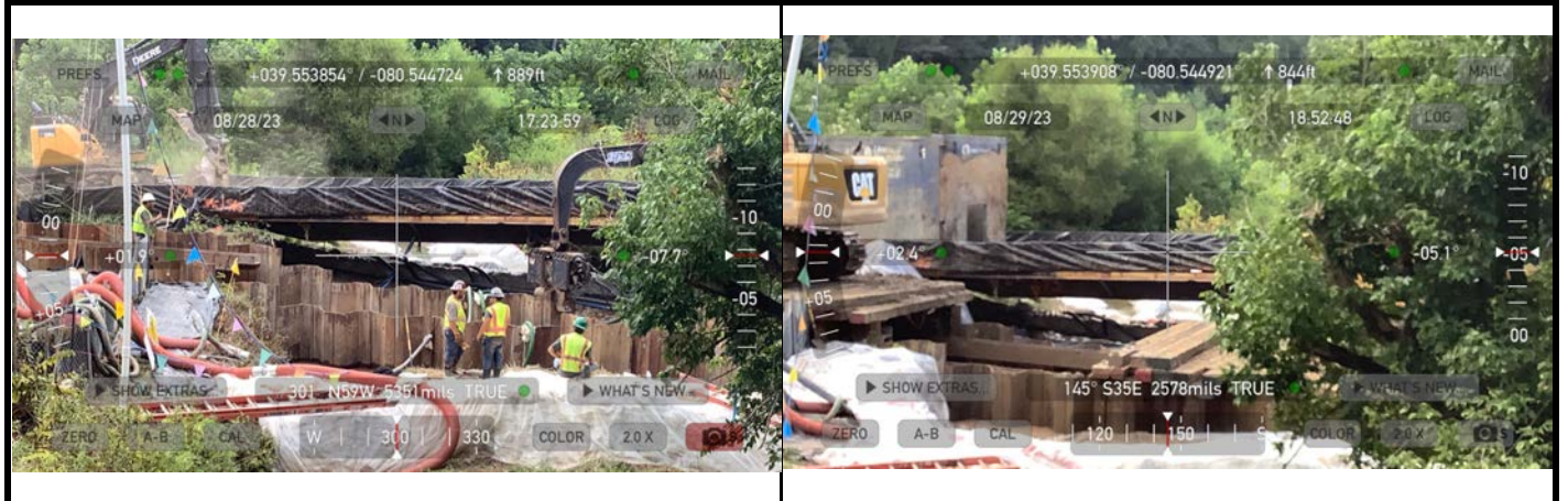
GPS Location See above. GPS Location See above. Description This photo shows the contractor continuing working on sheet piling installation. Description This photo shows the contractor continuing working on sheet piling installation.
