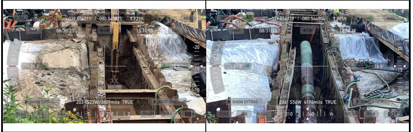
GPS Location See above. GPS Location See above. Description This photo shows the contractor working on trench excavation. Description This photo shows the contractor working on installing the pipe.
