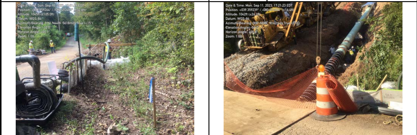
GPS Location Refer to photograph. GPS Location Refer to photograph. Description The dam and pump were prepared as excavation through crossing began. Description The pipe was lowered into the crossing.
