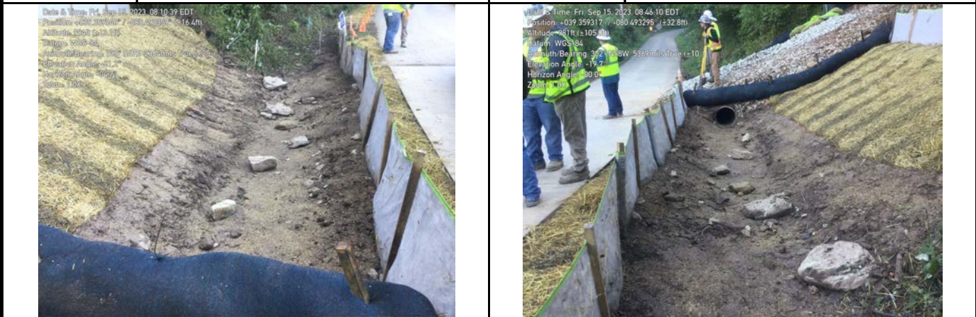
GPS Location Refer to photograph. GPS Location Refer to photograph. Description Downstream view of permitted impact area during post-construction assessment. Description Downstream view of unimpacted area during post-construction assessment.
