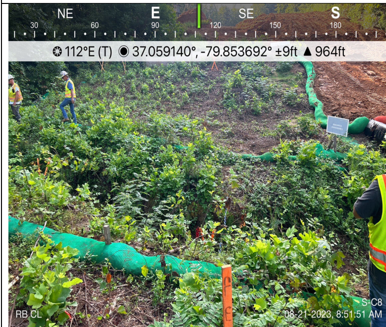
Photo Description: Pipe centerline view of the resource from the right bank prior to construction.
