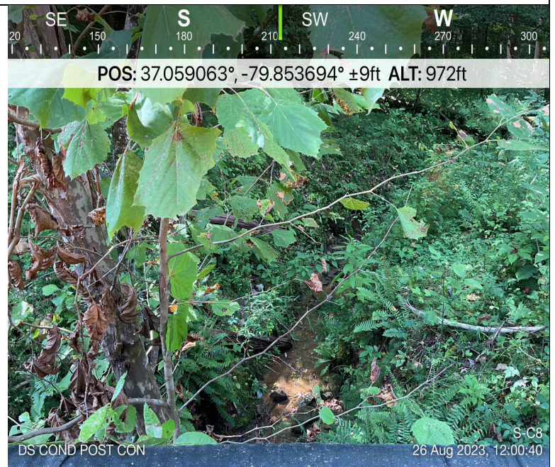
Photo Description: Downstream view of unpermitted area during post-construction assessment.
