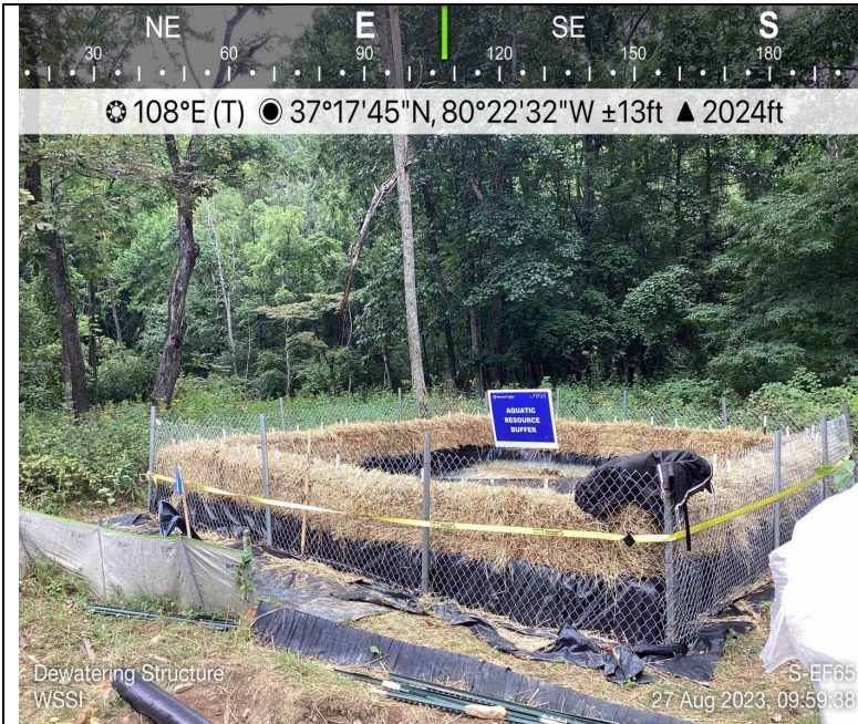
Photo Description: Dewatering structure located off ROW with landowner permission.
