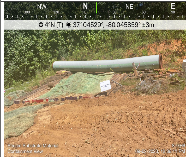
Photo Description: Stream substrate material contained with straw matting to prevent contamination.
