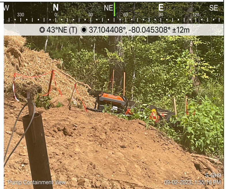
Photo Description: Pump containment structure to contain any potential leaks/spills.
