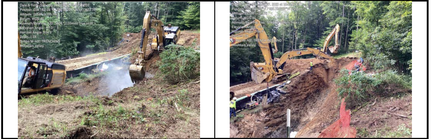
GPS Location See Photo GPS Location See Photo Description Photo 3: Trenching through wetland and stream. Description Photo 4: Lowering bedding into trench to prepare for pipe.
