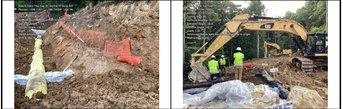
GPS Location See Photo GPS Location See Photo Description Photo 5: Trench breaks in place around resource (in background). Description Photo 6: Remove segregated material.
