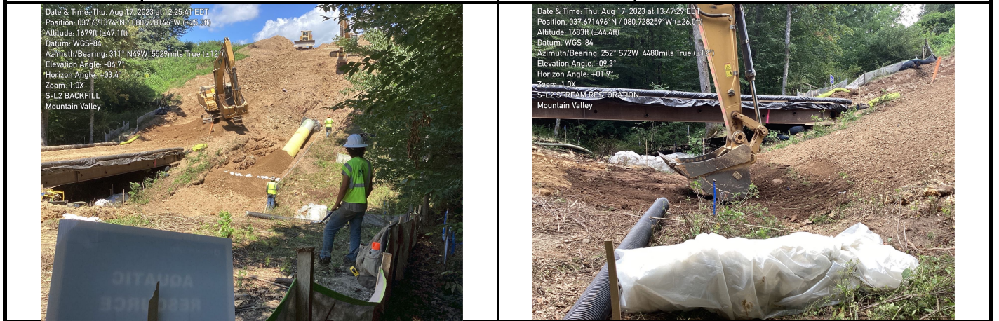
GPS Location Refer to Photo GPS Location Refer to Photo Description Photo 7. Trench backfill. Description Photo 8. Restoring stream topsoil.
