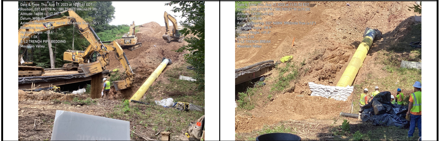
GPS Location Refer to Photo GPS Location Refer to Photo Description Photo 5. Placing bedding and backfilling. Description Photo 6. Trench breakers
