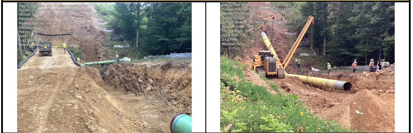
GPS Location Refer to Photo GPS Location Refer to Photo Description Photo 3. Trench through resource. Description Photo 4. Pipe lowered into resource.
