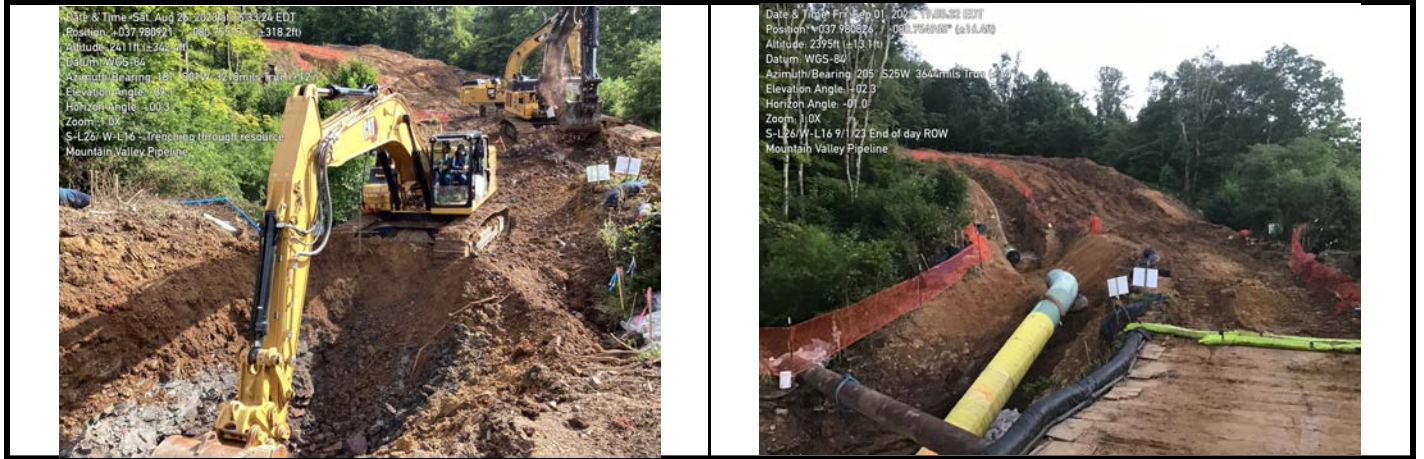
GPS Location See Photo GPS Location See Photo Description Photo 3: Trenching through aquatic resources. Description Photo 4: Pipe lowered into aquatic resources
