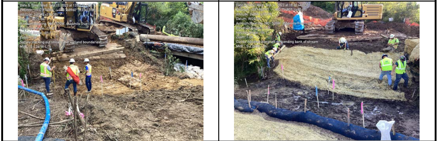
GPS Location See Photo GPS Location See Photo Description Photo 7: Survey staking out aquatic resources. Description Photo 8: Installing Curlex.
