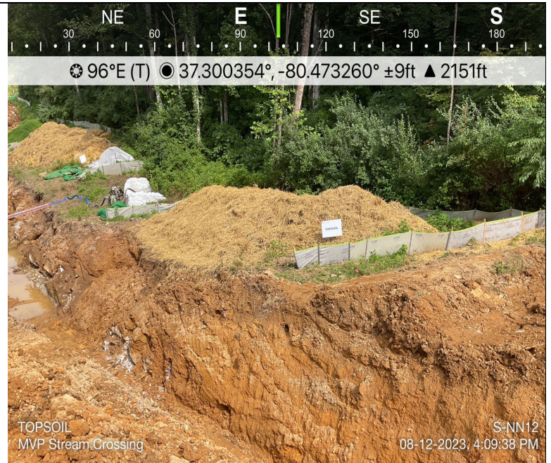
Photo Description: Segregation of soil.
