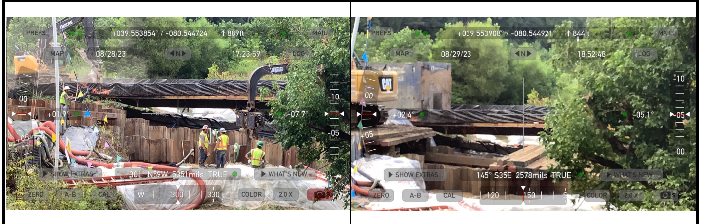
GPS Location See above. GPS Location See above. Description This photo shows the contractor continuing work on the sheet pile installation. Description This photo shows the contractor continuing work on the sheet pile installation.
