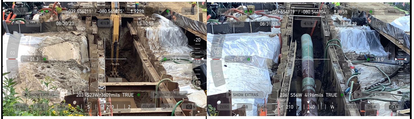
GPS Location See above. GPS Location See above. Description This photo shows the contractor working on excavating the trench Description This photo shows the contractor working on installation of pipeline.
