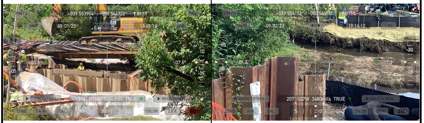
GPS Location See above. GPS Location See above. Description This photo shows the contractor working on backfilling the trench with soil. Description This photo shows the completed crossing.
