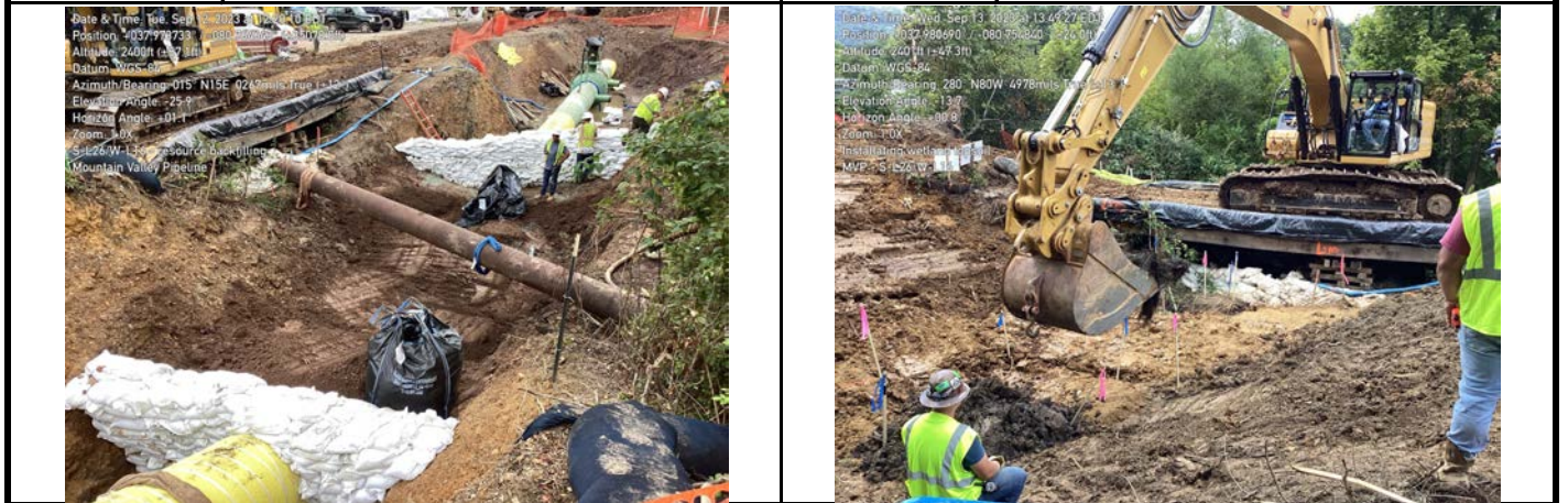
GPS Location See Photo GPS Location See Photo Description Photo 5: Constructing trench breaks. Description Photo 6: Restoring Wetland Soil.
