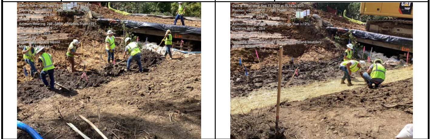
GPS Location See Photo GPS Location See Photo Description Photo 7: Distributing wetland soil by hand. Description Photo 8: Installing Curlex.
