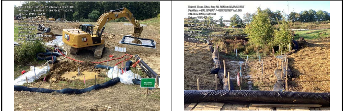
GPS Location See Photo GPS Location See Photo Description Photo 7: Stream substrate removed and segregated (9/19/2023). Description Photo 8: Stream surveyed and restored (9/20/2023).
