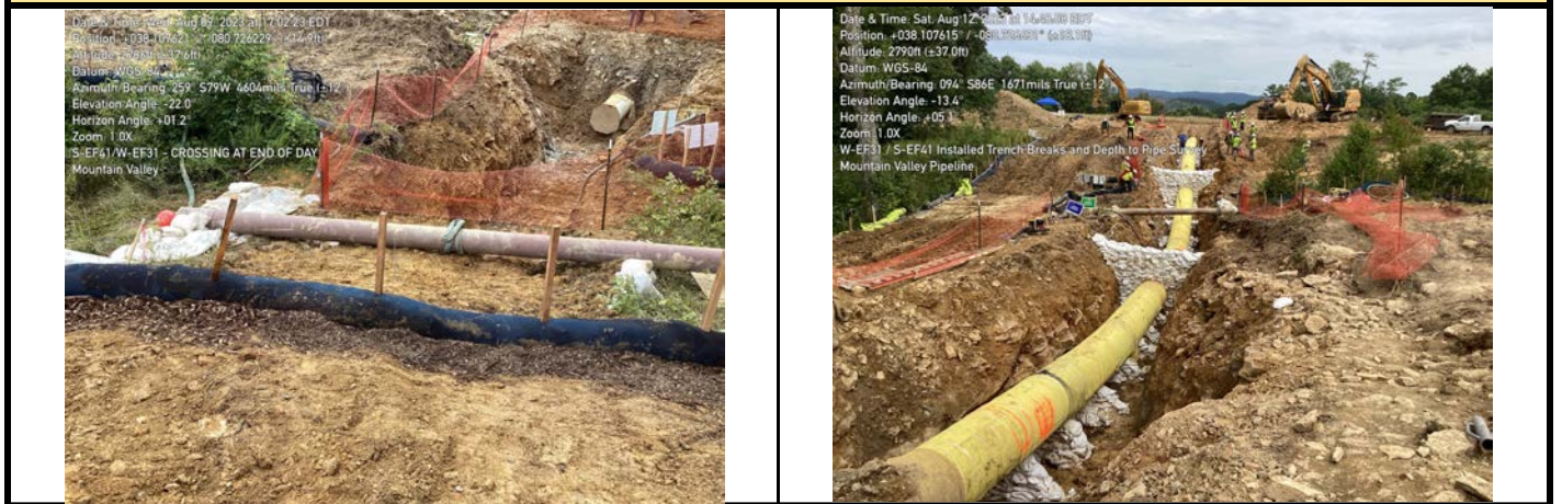
GPS Location See Photo GPS Location See Photo Description Photo 3: Trench on LDB Description Photo 4: Trench breaks installed.
