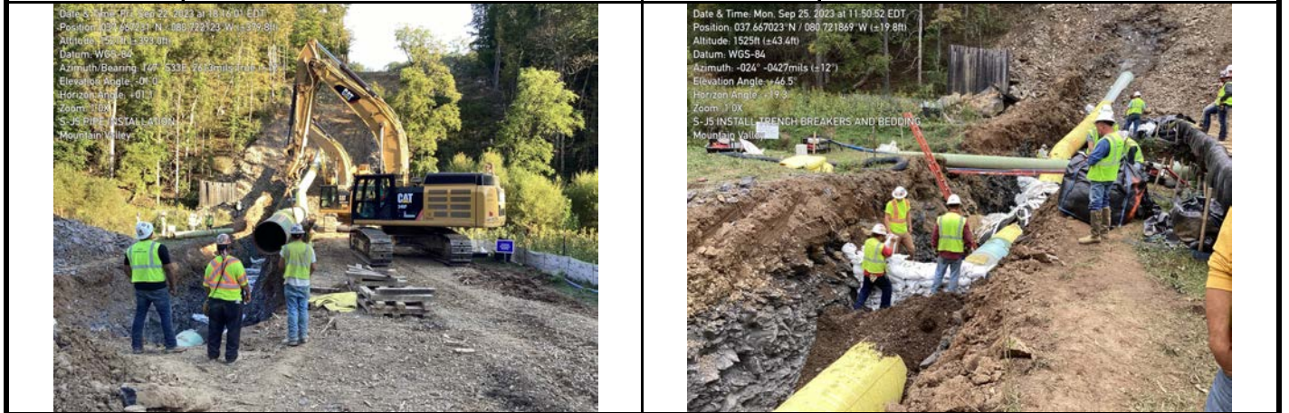
GPS Location See Photo GPS Location See Photo Description Photo 5: Lowering pipe into aquatic resource. Description Photo 6: River weights and trench breaks installed in aquatic resource area.
