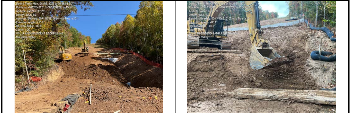
GPS Location See Photo GPS Location See Photo Description Photo 5: Trench breaker construction complete, backfilling of aquatic resource. Description Photo 6: Beginning restoration of aquatic resource.
