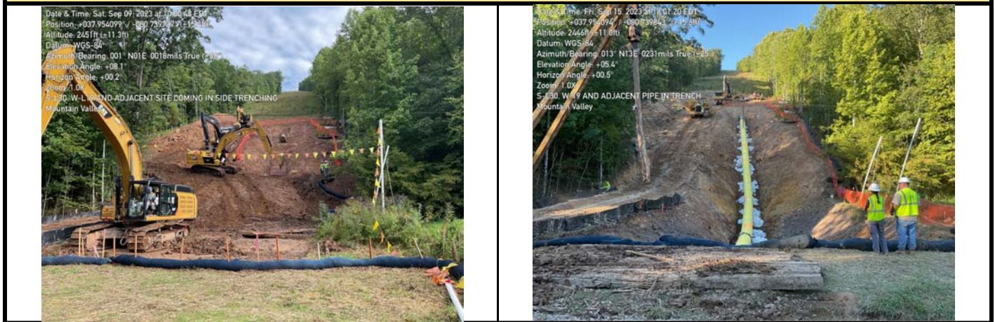
GPS Location See Photo GPS Location See Photo Description Photo 3: Excavation of trench in aquatic resource. Description Photo 4: Pipe placed into trench in aquatic resource lined with bedding.
