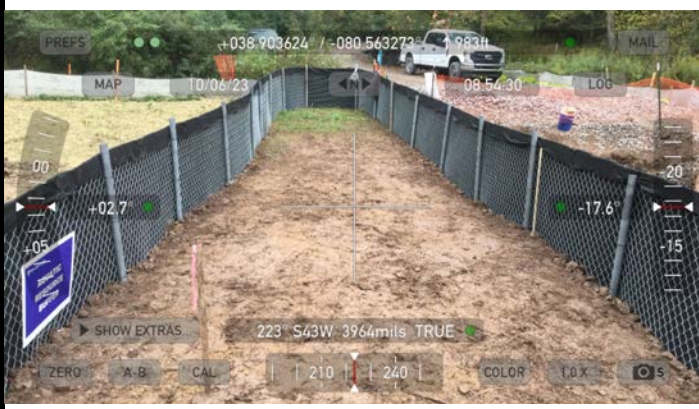
GPS Location See photo Description View of permitted resource impact area during post-construction assessment.
