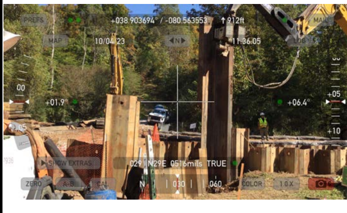
GPS Location See photo Description This photo shows the contractor removing the sheet piling from the wetland
