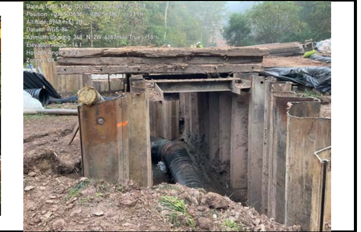
GPS Location See photo Description This photo shows the pipe installed in the wetland
