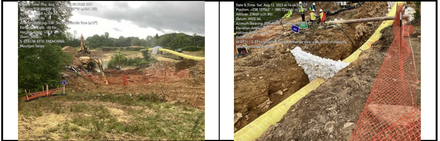
GPS Location See Photo GPS Location See Photo Description Photo 3. Excavating trench at crossing. Description Photo 4: Trench Breakers
