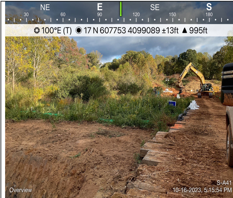
Photo Description: An overview of the pre-construction stream conditions. Bell hole excavation outside resource area.
