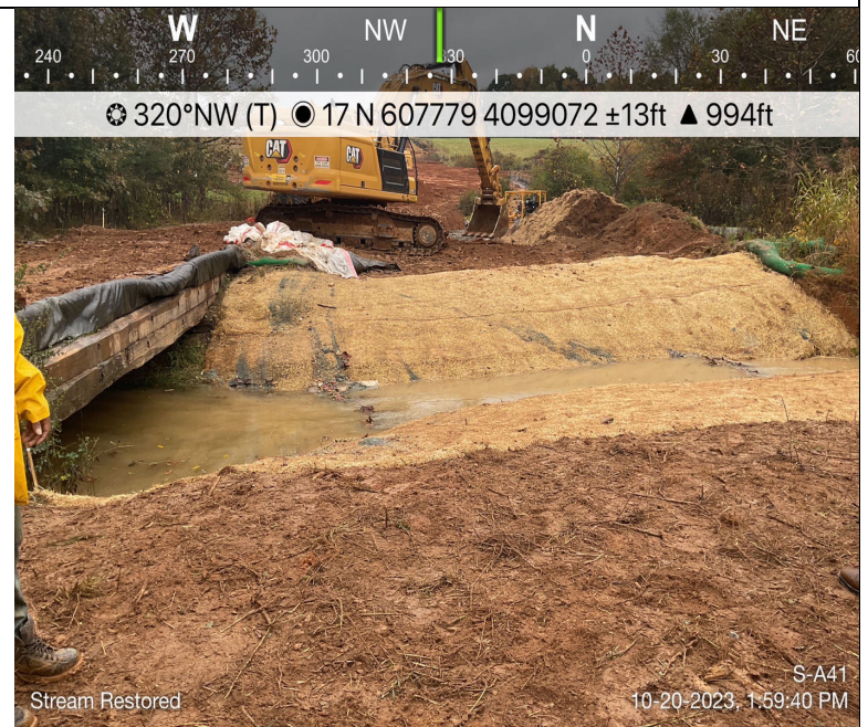
Photo Description: Flow restored to stream after the conclusion of restoration activities. Rock check dams remain installed across channel in attempt to control turbidity.
