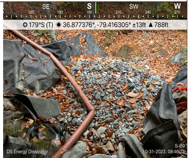
Photo Description: The energy dissipater for pump around operation.
