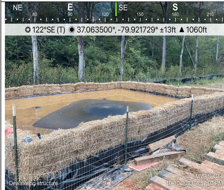
Photo Description: Dewatering structure
