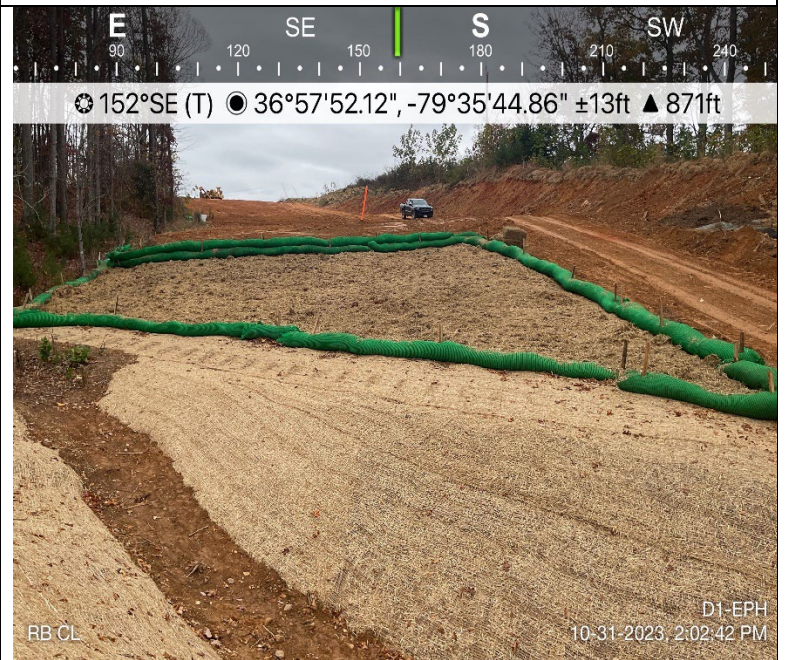
Photo Description: The site after the application of seed and erosion control matting.
