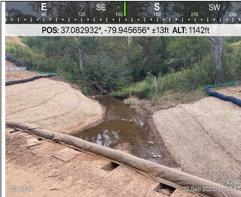
Photo Description: Downstream view of restoration 5 days post-restoration. No accumulated material, significant turbidity, or signs of accelerated erosion of stream banks was observed.
