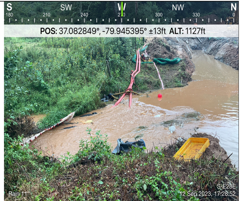
Photo Description: Open trench flooded and downstream dam overtopped by rain/flood waters.
