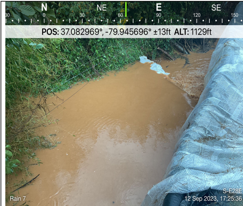
Photo Description: Overtopped/flooded upstream dam at S-E28-E crossing.
