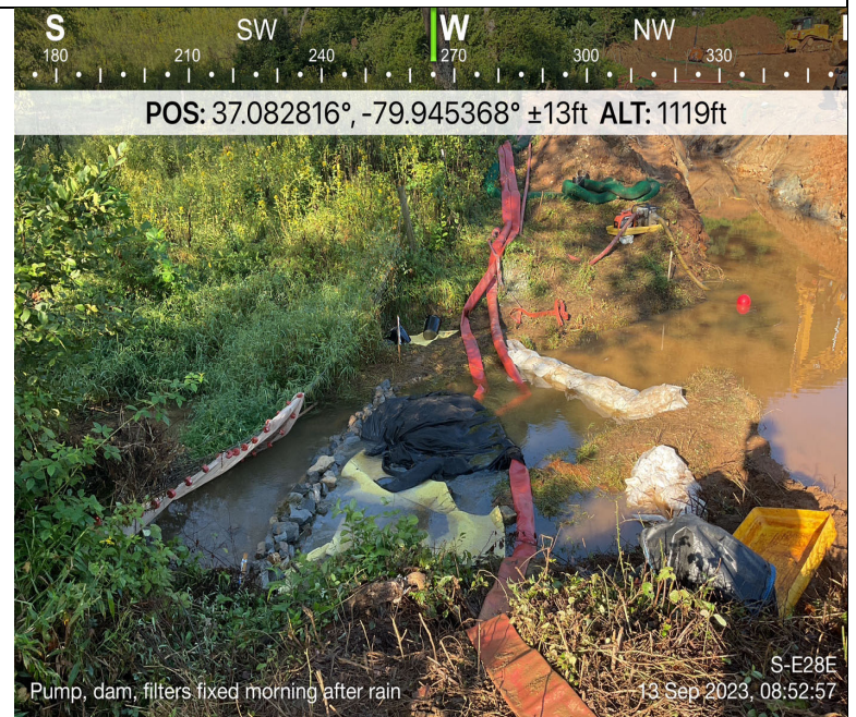
Photo Description: Downstream dam re-established and flooded trench now isolated from S-E28-E stream flow. Downstream turbidity significantly reduced from work area turbidity.
