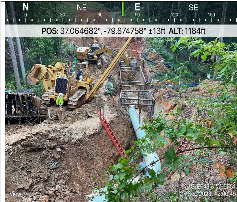
Photo Description: Pipe lowered into trench and trench boxes installed for safety.
