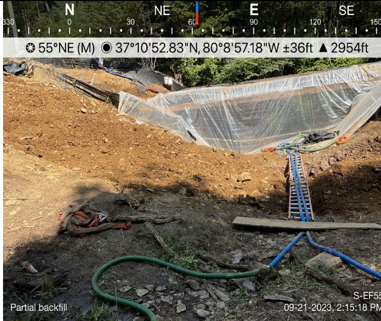
Photo Description: Partial backfill of resource with subsoil prior to restoration. Dam and pumps remain installed and functioning.
