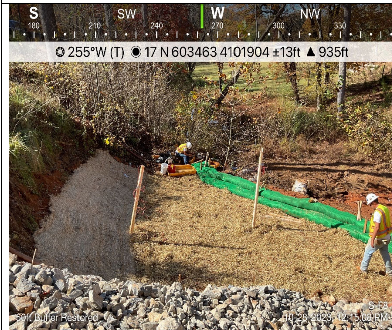
Photo Description: Restoration of the 50-foot buffer. Modification to right bank to account for step/eroded stream bank.
