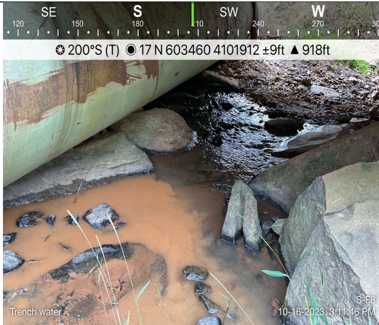
Photo Description: Turbid water emerged from stream bank during excavation of pipe loose ends in upland area.
