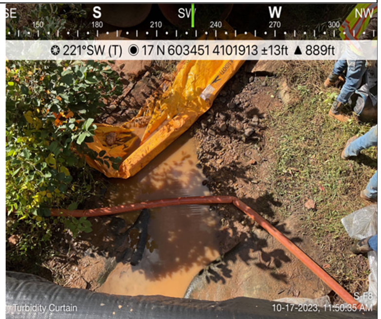
Photo Description: Turbidity curtain installed to control turbidity from entering the resource during trench pump-down.
