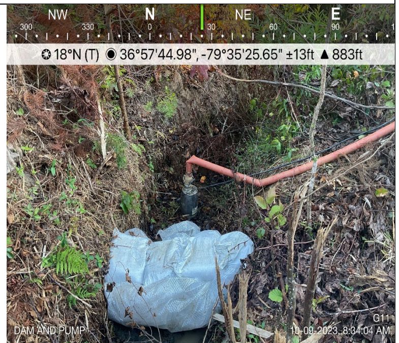
Photo Description: Dam and pump around crossing installed and functional throughout crossing activity.
