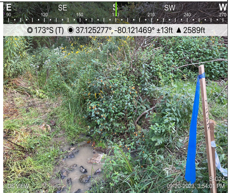
Photo Description: Conditions of the downstream area outside the ROW during post-construction assessment. Typo in photo, "DS COND", not DS VIEW.
