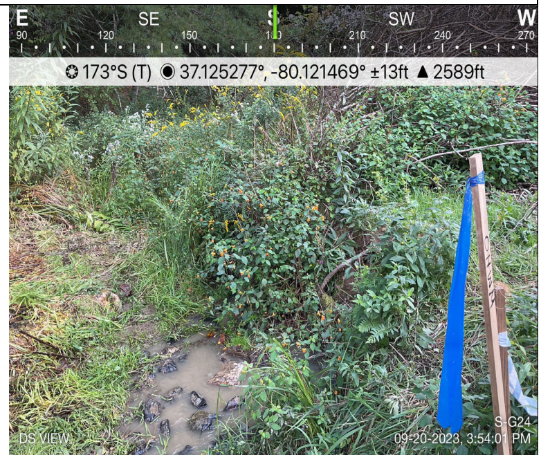
Photo Description: Conditions of the downstream area outside the ROW during post-construction assessment. S-G25 converges with S-G24 within the impact area, which then flows off the ROW. Typo in photo, "DS COND", not DS VIEW.
