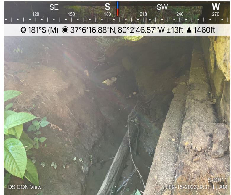
Photo Description: Conditions of the downstream area outside the ROW during pre-construction assessment.
