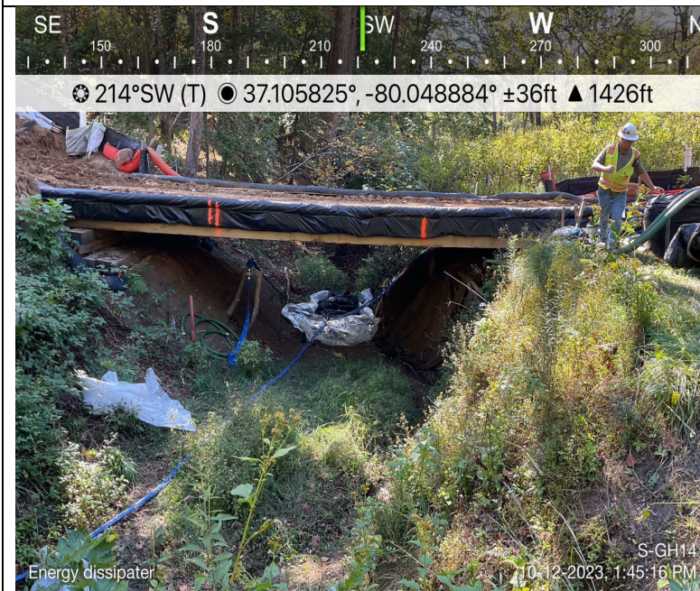
Photo Description: Energy dissipater.
