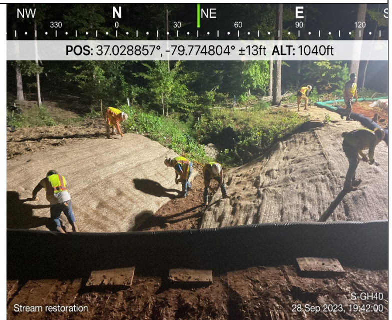
Photo Description: Restoration crews staking in erosion control matting along the streambanks.
