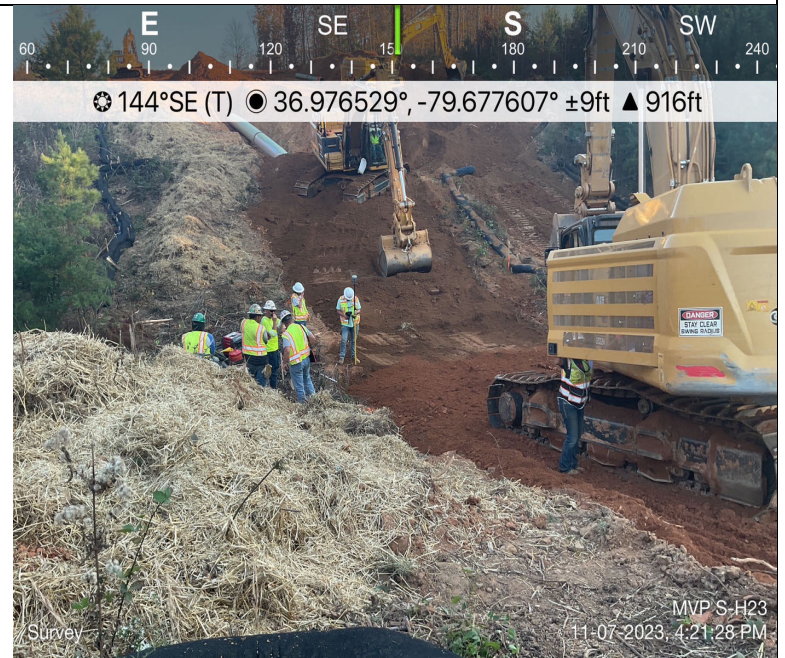
Photo Description: The survey crew taking elevations which were used during reconstruction.
