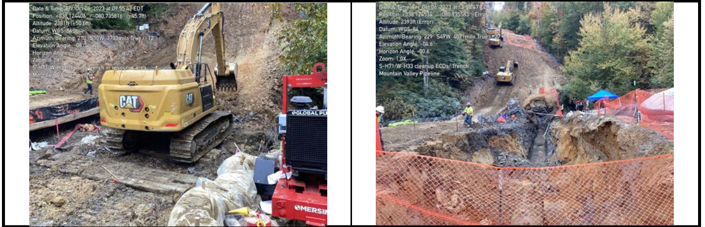
GPS Location See Photo GPS Location See Photo Description Photo 3: Begin trenching in resource area. Description Photo 4: Trench through resource area.
