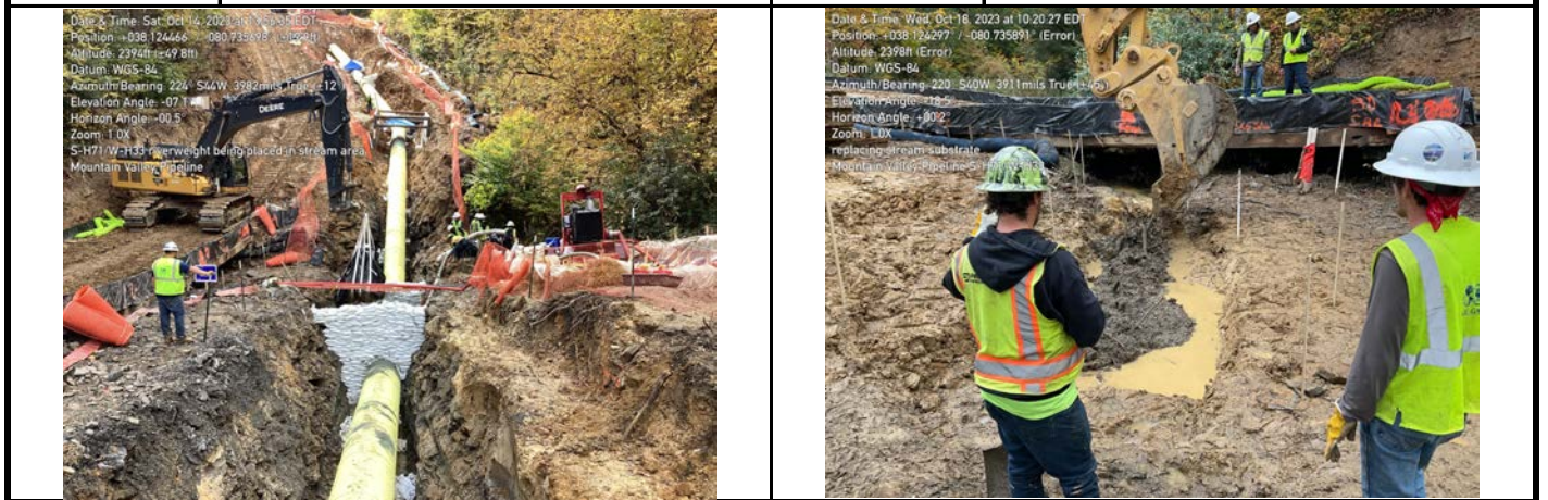
GPS Location See Photo GPS Location See Photo Description Photo 7: Placement of river weights in resource area. Description Photo 8: Restoring stream substrate.
