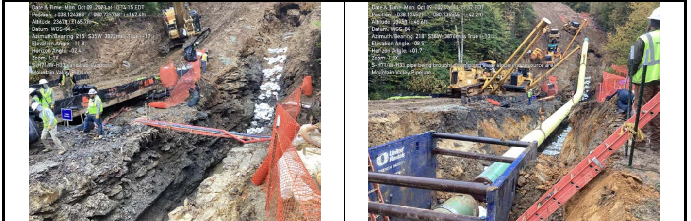
GPS Location See Photo GPS Location See Photo Description Photo 5: Padding placed in trench. Description Photo 6: Placing pipe in resource area.
