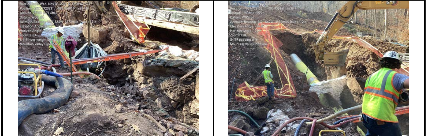
GPS Location See Photo GPS Location See Photo Description Photo 5: Constructing trench breakers and adding river weights in aquatic resource area. Description Photo 6: Sifting padding dirt in aquatic resource area.
