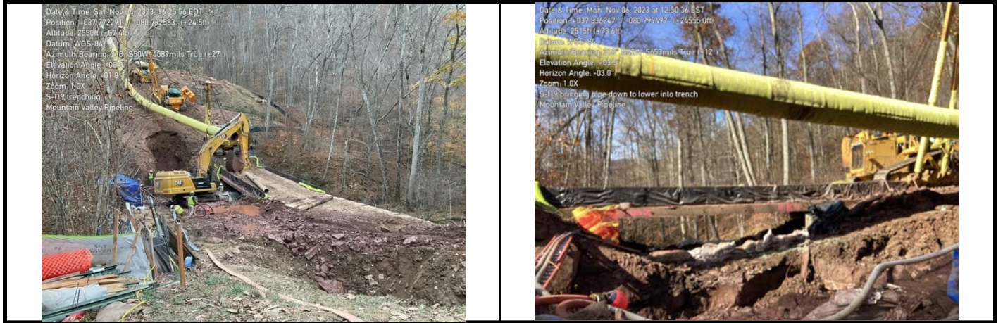
GPS Location See Photo GPS Location See Photo Description Photo 3: Trenching through aquatic resource area. Description Photo 4: Lowering pipe into trench.
