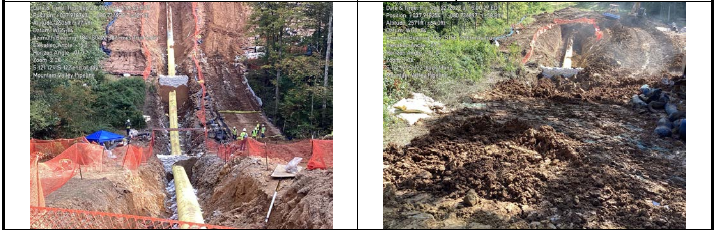
GPS Location See photo GPS Location See photo Description Photo 5: Trench breakers both sides of aquatic resources. Description Photo 6: Backfilling of aquatic resources.
