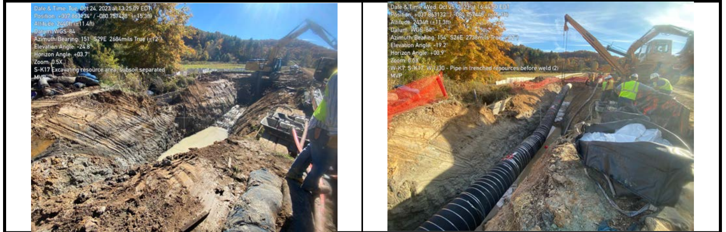
GPS Location See Photo GPS Location See Photo Description Photo 3: Excavating through aquatic resource and upland area. Description Photo 4: Staging of pipe through aquatic resource.
