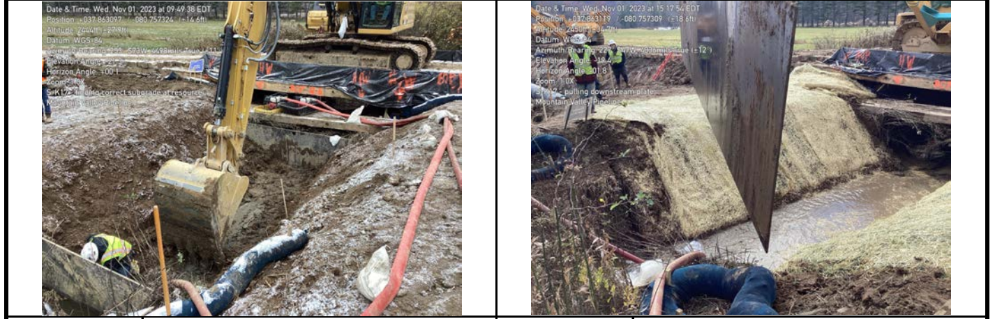
GPS Location See Photo GPS Location See Photo Description Photo 7. Contouring and achieving correct subgrade. Description Photo 8. Removing of steel plates and restoring flow.
