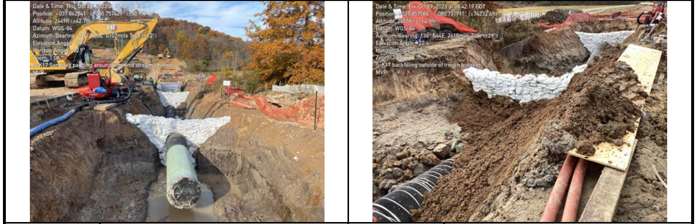
GPS Location See Photo GPS Location See Photo Description Photo 5: Trench breakers being constructed around aquatic resource. Description Photo 6: Filling trench.
