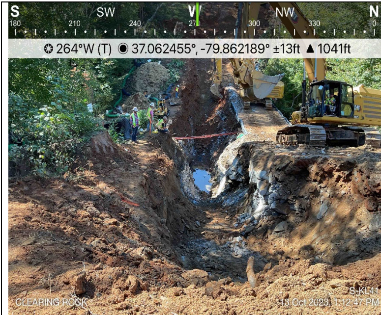
Photo Description: Rock excavation of trench. Dam and pump functional and hoses conveyed across trench via extension ladder.
