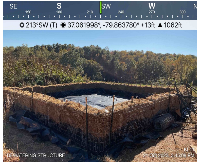
Photo Description: Dewatering structure installed and available for use throughout crossing activity.
