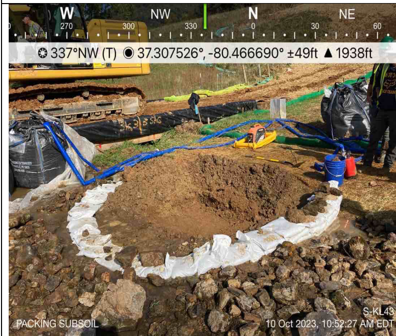
Photo Description: Subsoil compacted in subsidence.
