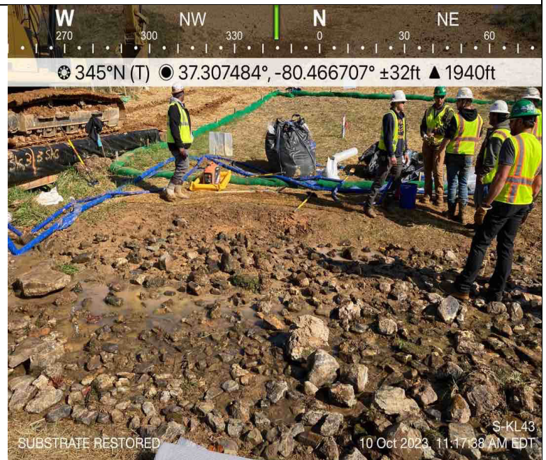
Photo Description: Substrate and stream restored. Cofferdam removed from around subsidence remediation area.
