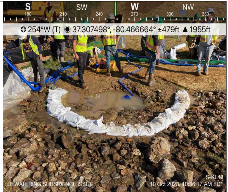
Photo Description: Subsidence issue area being dewatered prior to repairs.
