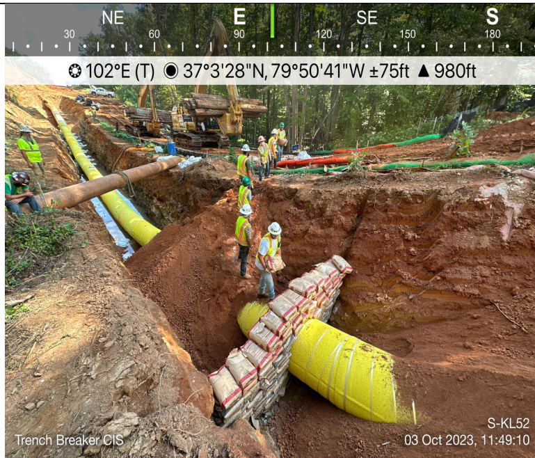
Photo Description: Trench breaker installation on coming in side of stream resource. Flume remained installed during crossing activities.
