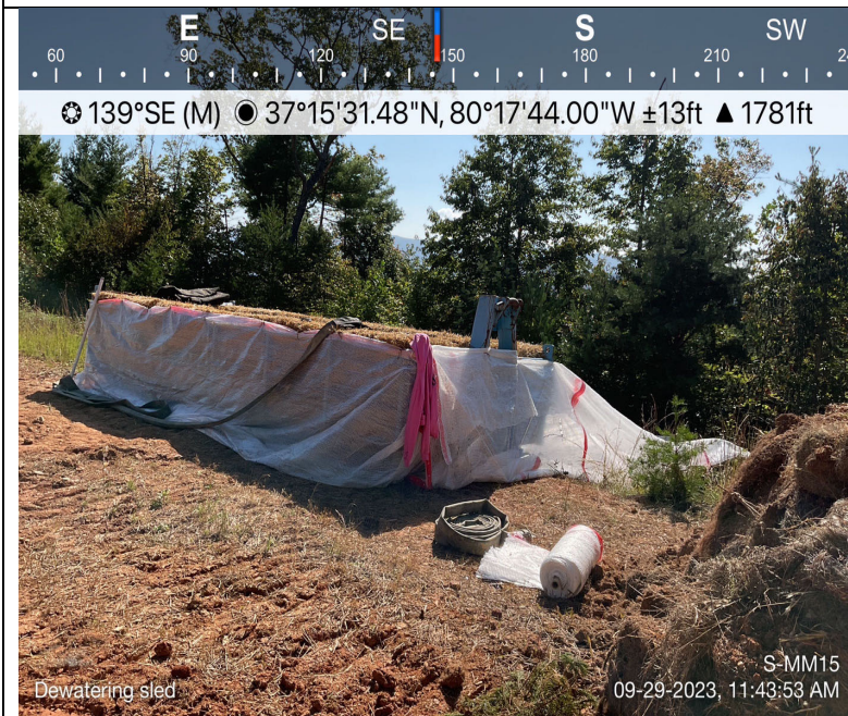
Photo Description: Dewatering sled.
