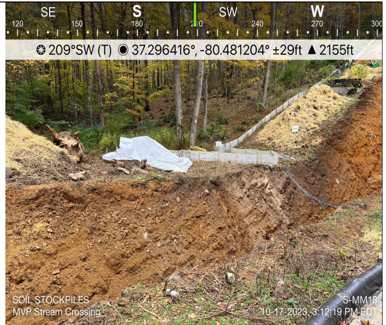
Photo Description: Topsoil and stream substrate stockpiles. Dam and pump installed for conveyance for stream flow, if needed.
