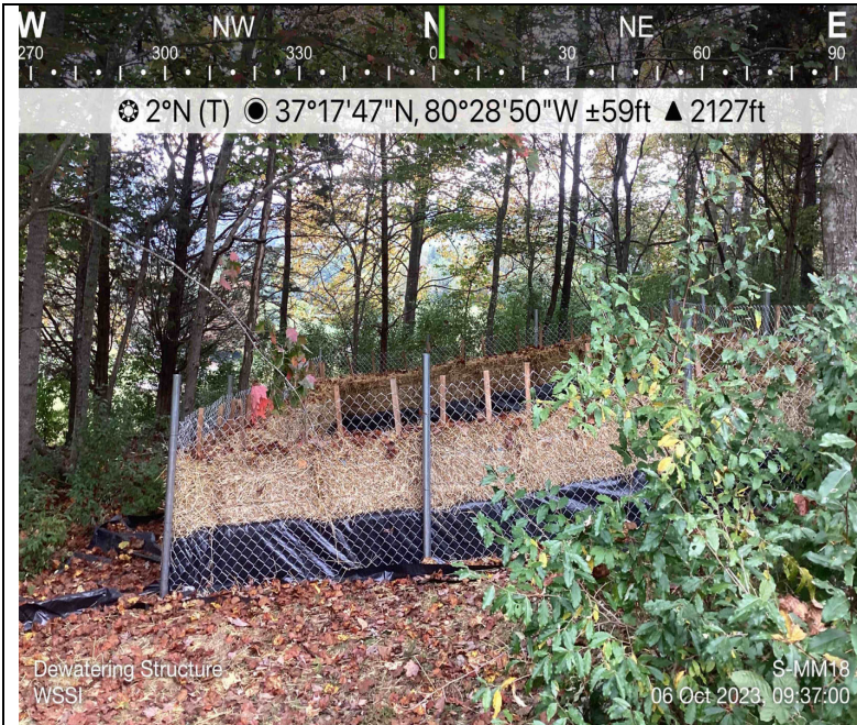
Photo Description: Dewatering structure located off of the LOD with project permissions.
