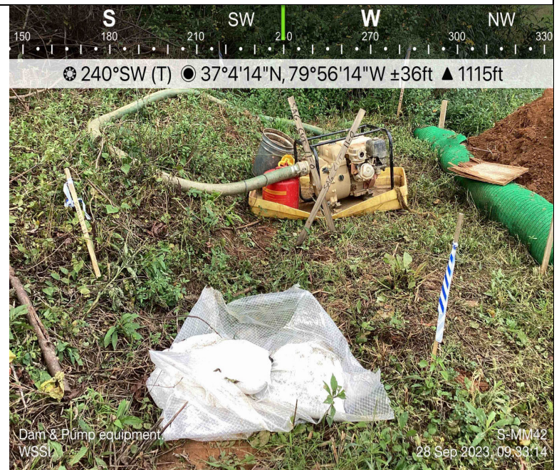
Photo Description: Dam and pump materials installed for crossing. Resource was dry during crossings, and pump arrounds were not needed to convey water around workspace.
