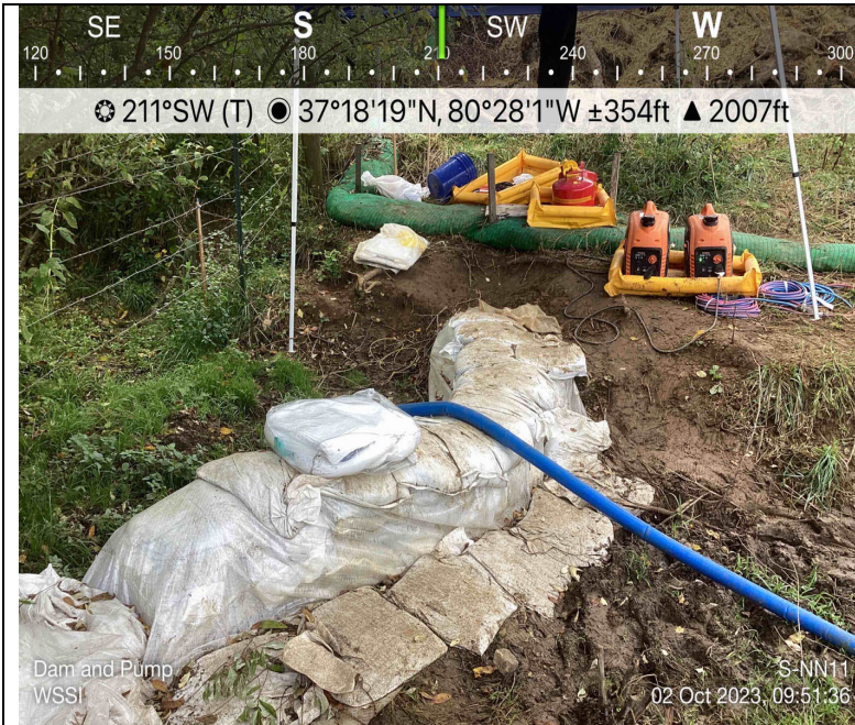
Photo Description: Dam and pumps installed and functioning.
