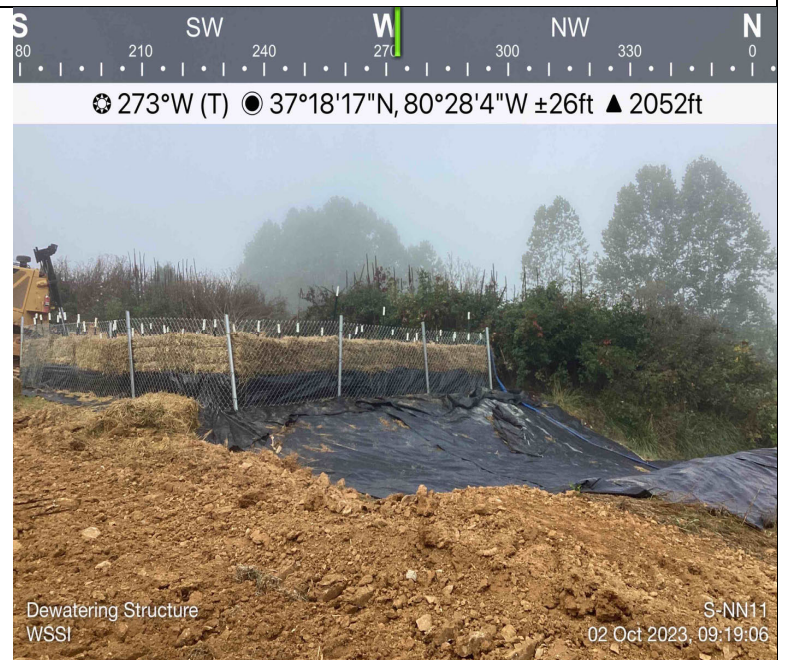
Photo Description: Dewatering structure located on-site.
