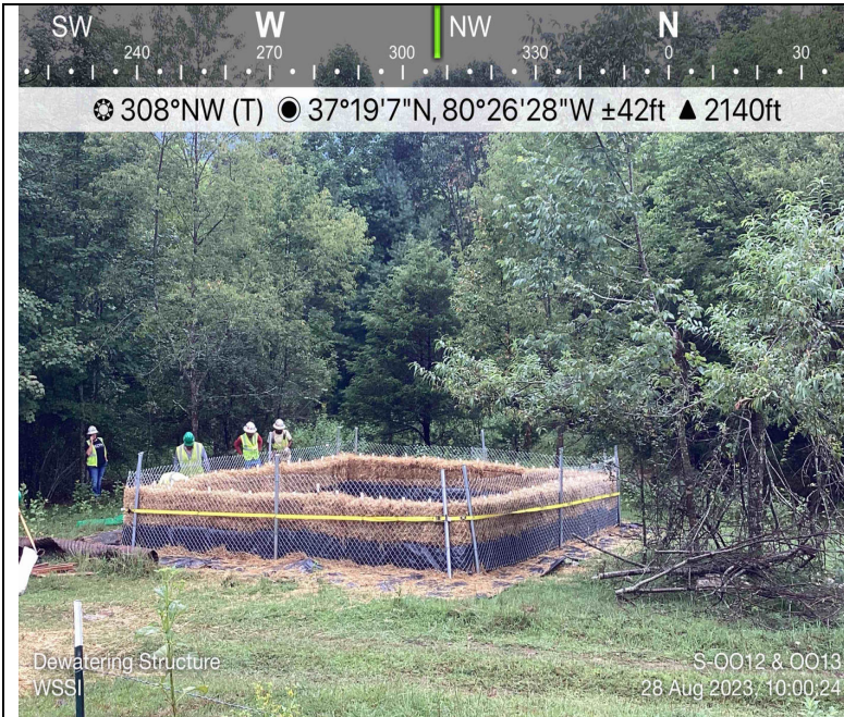
Photo Description: Dewatering structure located off ROW with landowner permission and shared with OO12.
