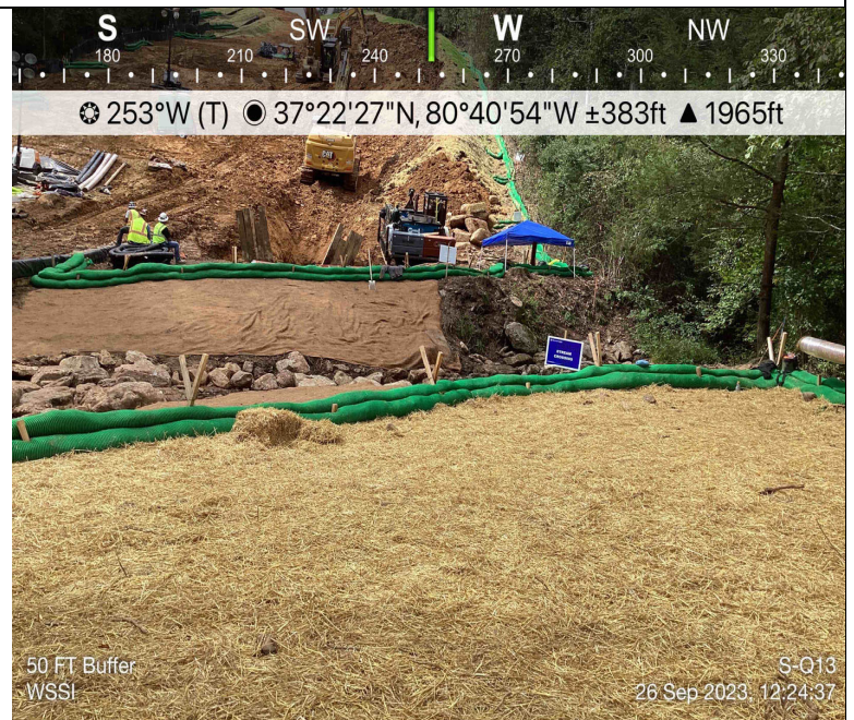
Photo Description: 50' buffer restored on right side with left side left open for tie in.
