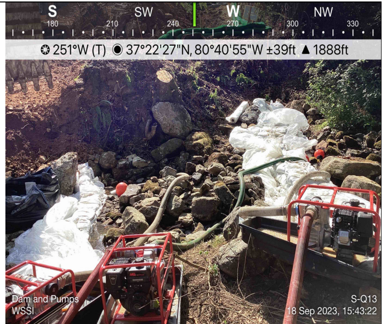
Photo Description: Double dam and pump around due to poor sealing.
